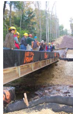
DCNR Asst. District Forester Joe Dotzel describes how a gas pipeline was installed to cross a stream within the State Forest.
